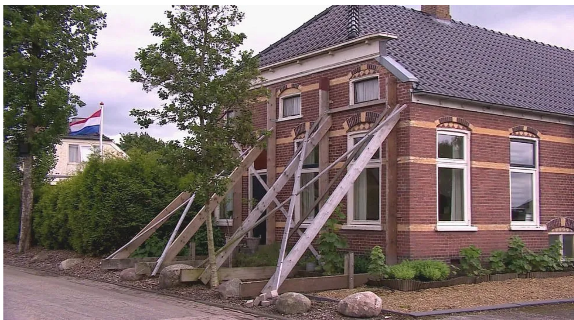
Figure 1: Reinforcement of some properties in Groningen due to earthquake risk, while others are deemed too dangerous to inhabit, illustrating the impact of induced seismic activity on local infrastructure.
